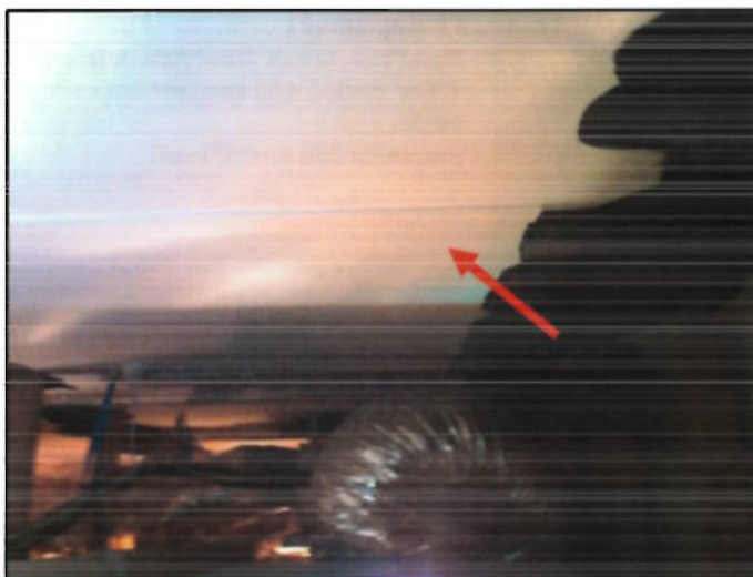
Photograph 18 Ground Floor, FCS ceiling sheeting within ceiling cavity (asbestos containing).
