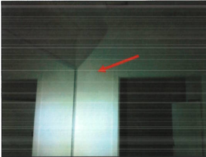
Photograph 16 Second Floor, Female Toilet Airlock Room, FCS wall sheeting (all walls) (asbestos containing).
