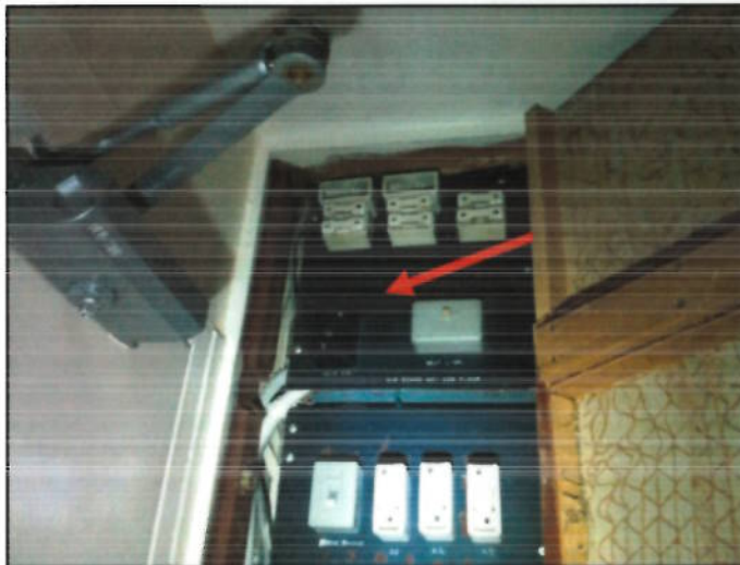
Photograph 11 Second Floor, Western Electrical Distribution Cupboard, upper BEBB (asbestos containing).
